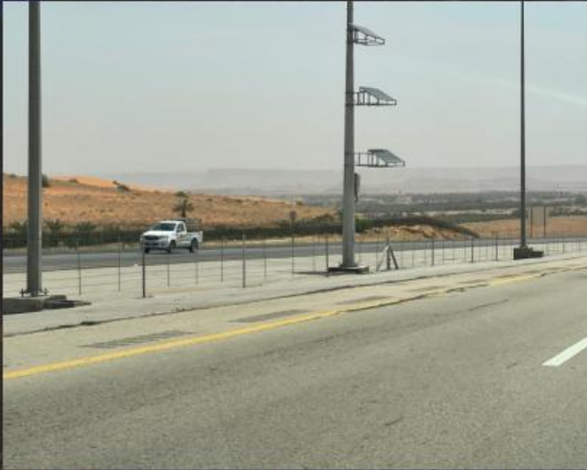
Lighting columns & CCTC
